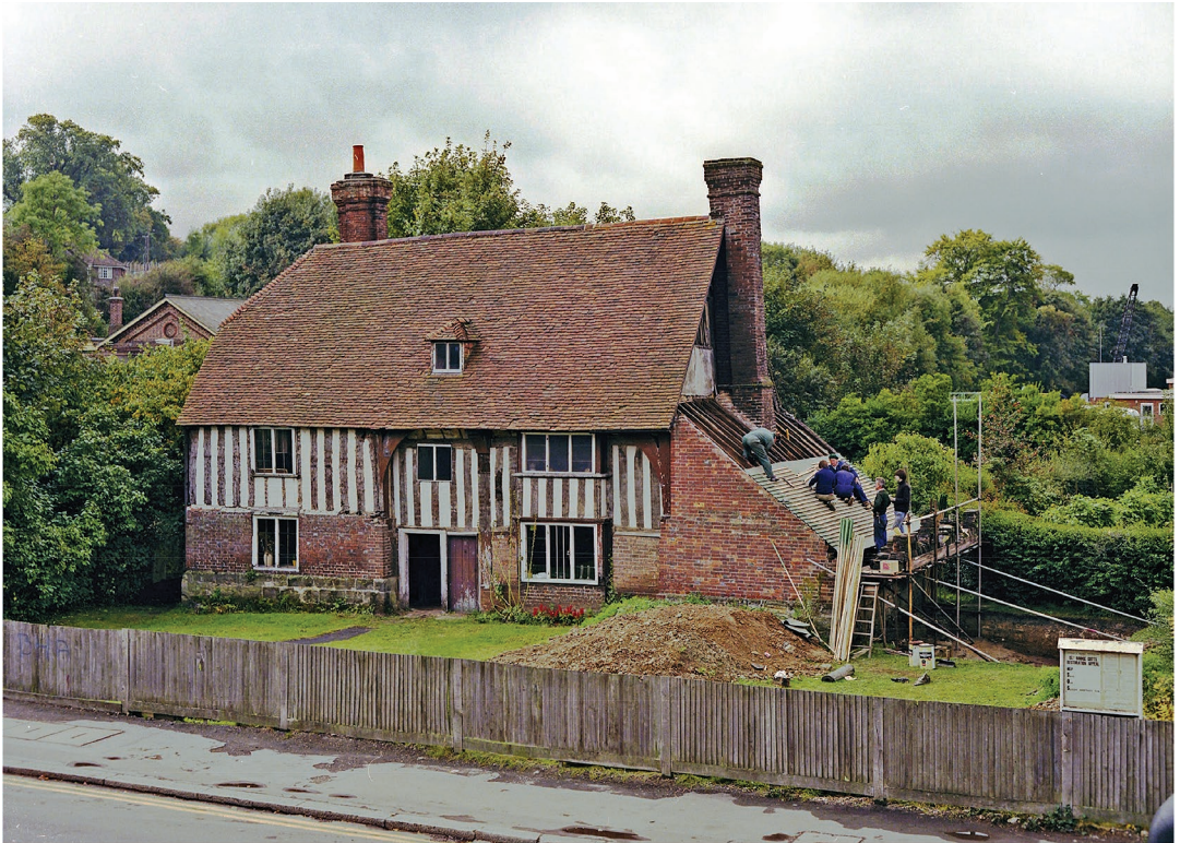
Fig. 24. Photo of Bridge Cottage prior to its renovation, showing how the building would have largely appeared in the early 18th century.
